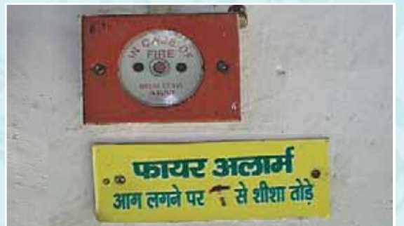
Emergency Fire Alarm Point
